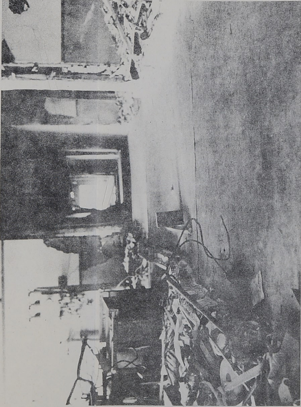
8. Dished concrete panels of the ground floor of the Administration Building in the Torpedo Factory at Nagasaki. The basement was practically air tight and was used as an air-raid shelter. Distance 4050 ft., peak pressure 10 p.s.i.
